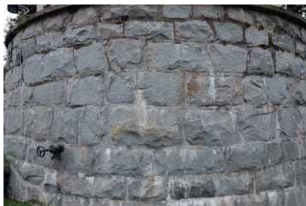
Fig. 14b. Dressed blocks of granodiorite used in the foundation for the Puijo Tower. (Photo: Jari Nenonen, GTK)
